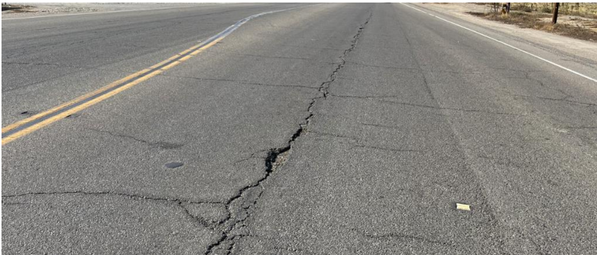
Figure 6. Typical pavement conditions – longitudinal cracking, transverse cracking
