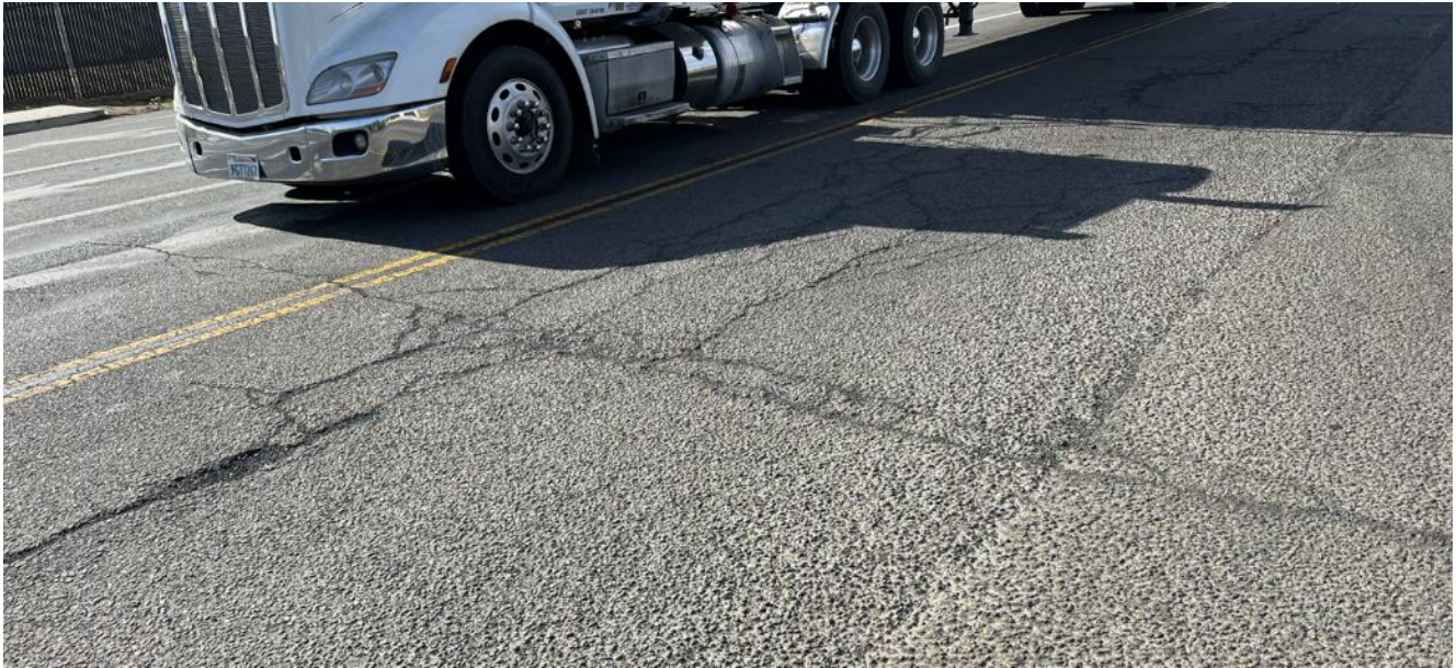
Figure 5. Typical pavement conditions – weathering and raveling and cracking
