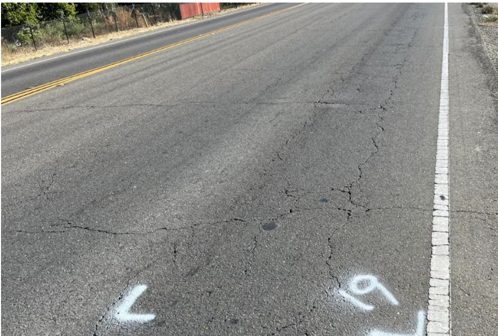
Figure 8. Typical pavement conditions – utility/block cracking, rutting - treated with base repairs
