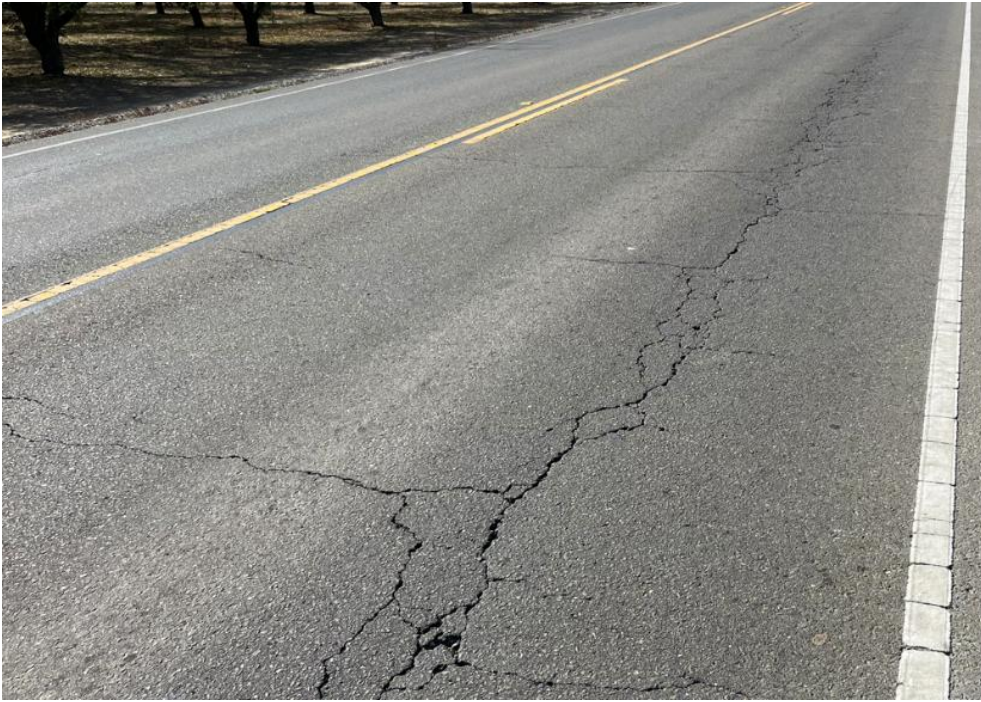
Figure 7. Typical pavement conditions – longitudinal cracking, medium alligator cracking
