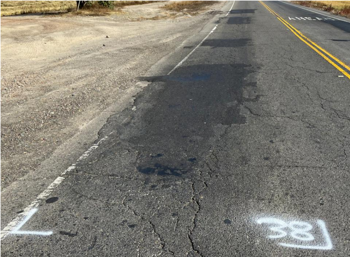
Figure 9. Typical pavement conditions – patching, rutting - treated with base repairs
