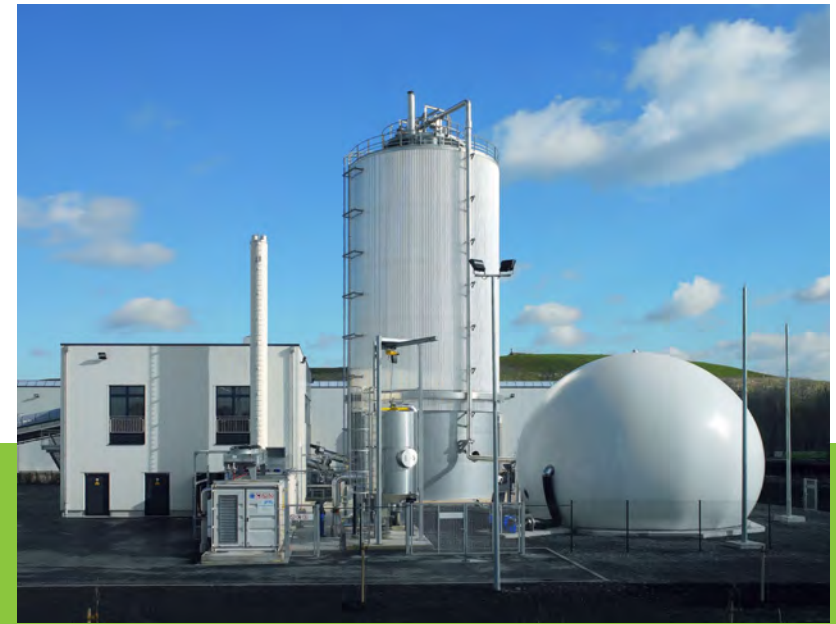
Organic Waste Systems Anaerobic Digestion Facility in Munster, Germany
