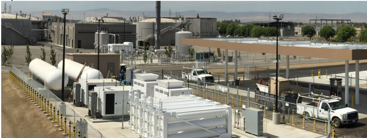
The city's new R-CNG Fueling Facility where the Waste to Fuel program will operate. Photo: City of Manteca
