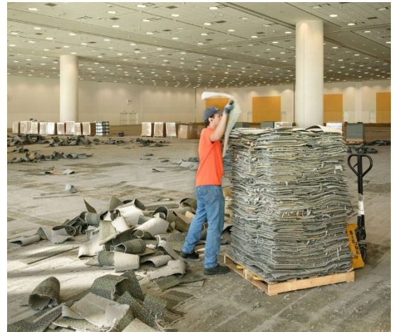
Tarkett staff stacking carpet tiles during renovation of Moscone Center in San Francisco.
