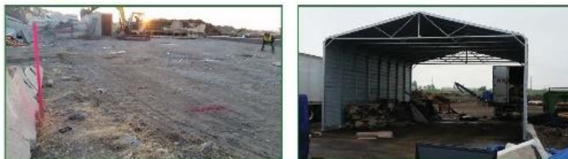
Zanker Recycling "before" (left) and "after" (right) with weather cover for carpet.
