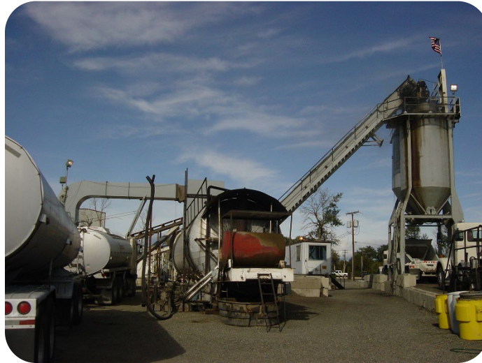
Figure 31. Asphalt binder storage tanks.
