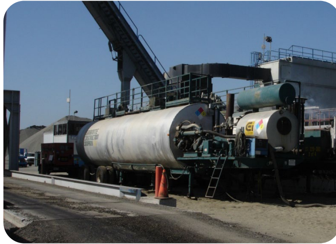
Figure 35. Asphalt rubber binder storage tank.
