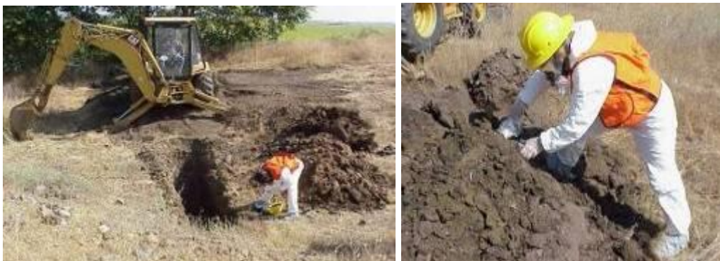
Figure 37: Farm-tractor backhoe conducts trenching; field staff document trench characteristics (length, depth, cover thickness, description of waste), perform instrument screening (combustible gas, oxygen levels, H 2 S) and also obtain samples for chemical and physical analysis.
