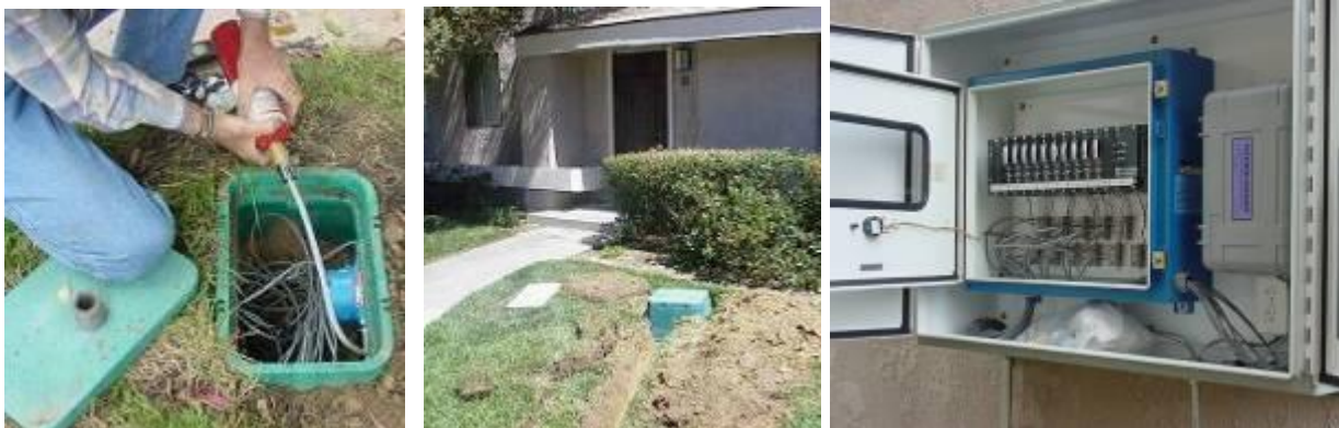
Figure 35: Subsurface vaults with combustible gas sensors are installed adjacent to the foundations of condominiums to detect and measure the concentration of methane gas migrating from the disposal area; a controller and data logger were used to collect gas measurements
