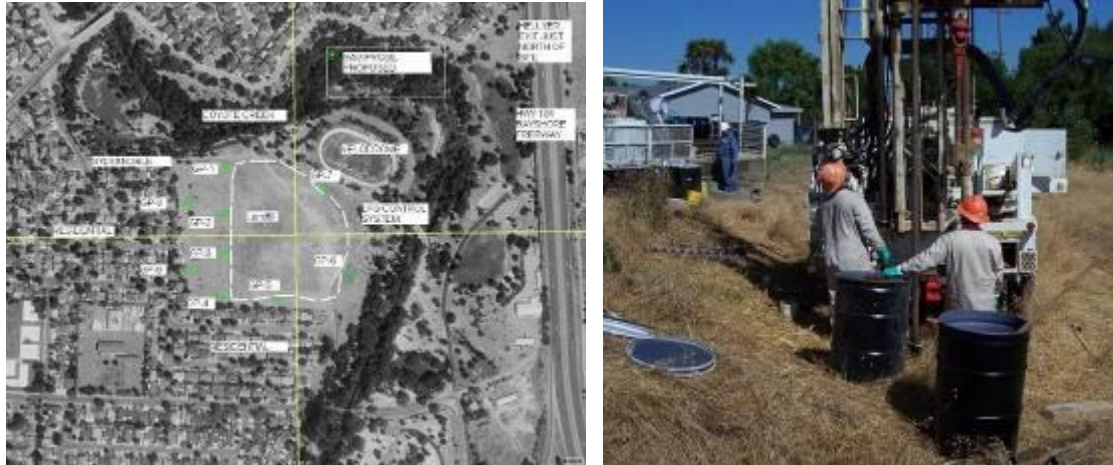
Figure 27: CIWMB designed and constructed a Landfill Gas Monitoring Network to determine if landfill gas migration was occurring into adjacent areas.
