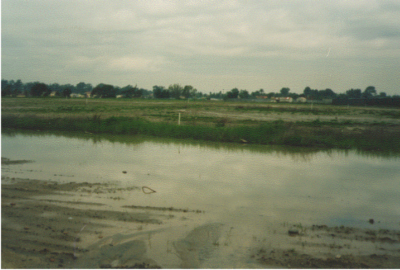
Figure 18 - Ponding on Landfill Surface
