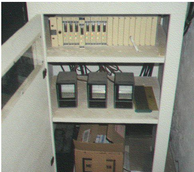
Figure 11 - Continuous Monitoring Equipment
