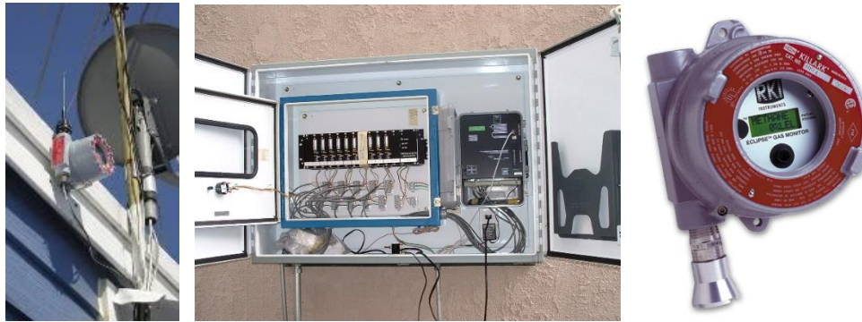
Figure 1. Continuous Gas Monitoring Equipment
