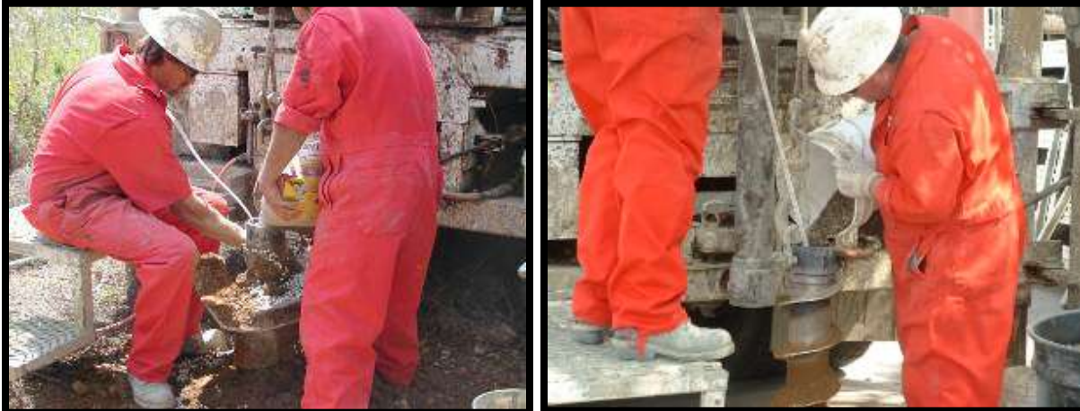
Figure 18: Drilling crew pouring bentonite pellets and constructing well-bore seal in annular space (following this process, water will be added to hydrate pellets); using tape to measure down-hole distance to start and finish of well-pack material (Monterey sand) for screened interval.
