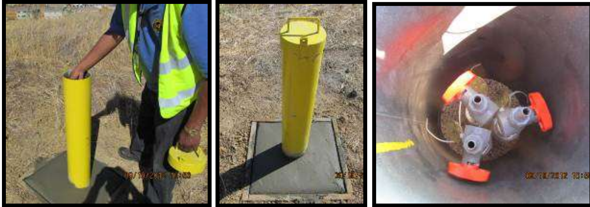
Figure 21: LFG monitoring well monument with locking well head cover – triple completion well with plastic lab cock valves
