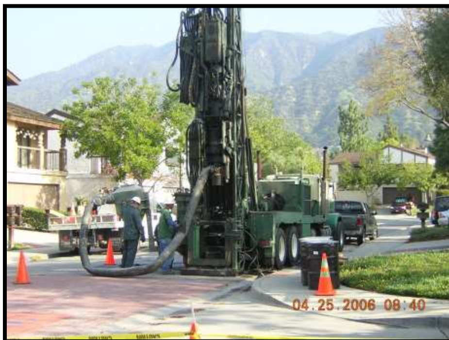
Figure 51: Landfill gas monitoring well construction in a residential area adjacent to the Canyon Park Landfill
