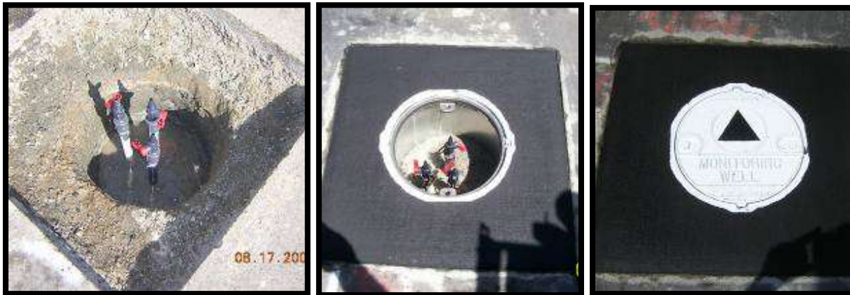
Figure 22: Flush-mounted LFG monitoring well with traffic-rated vault (LFG well in street)
