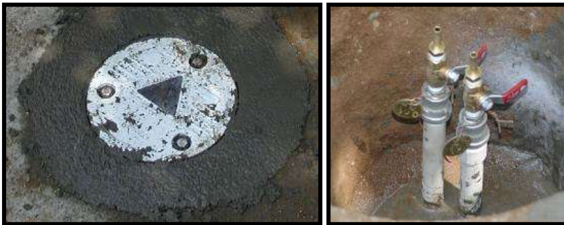
Figure 19: Flush-mounted LFG monitoring well with traffic-rated vault; dual completion well head with brass lab cock valve and brass identification tags (Probe ID & Depth)
