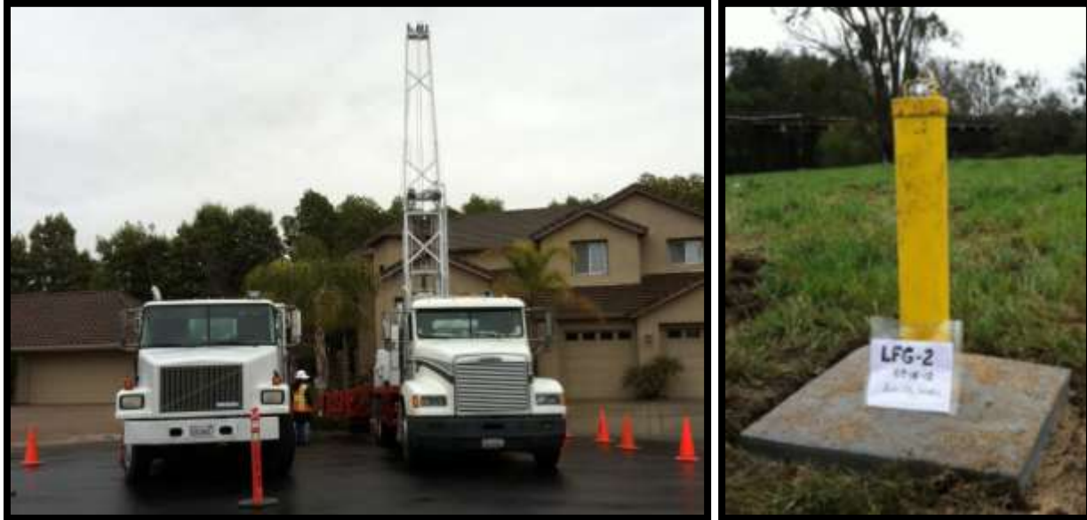
Figure 57: Landfill gas monitoring located near the south boundary of the landfill east of the railroad tracks; monitoring wells being constructed in a residential subdivision west of the railroad tracks
