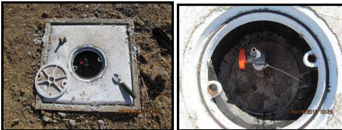
Figure 20: Flush-mounted vault in concrete pad in undeveloped area; single probe with plastic lab cock valve
