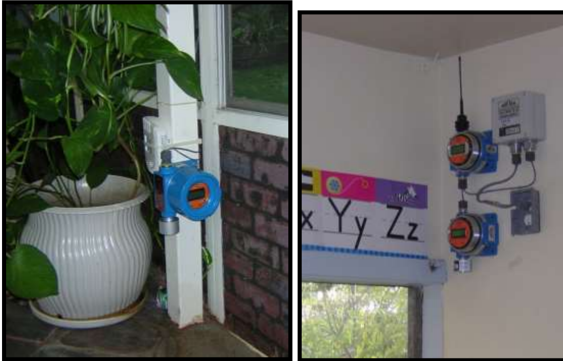
Figure 60: Infrared combustable gas sensor installed in the patio area of a residence; wireless transmitter and infrared sensor installed at the YMCA.
