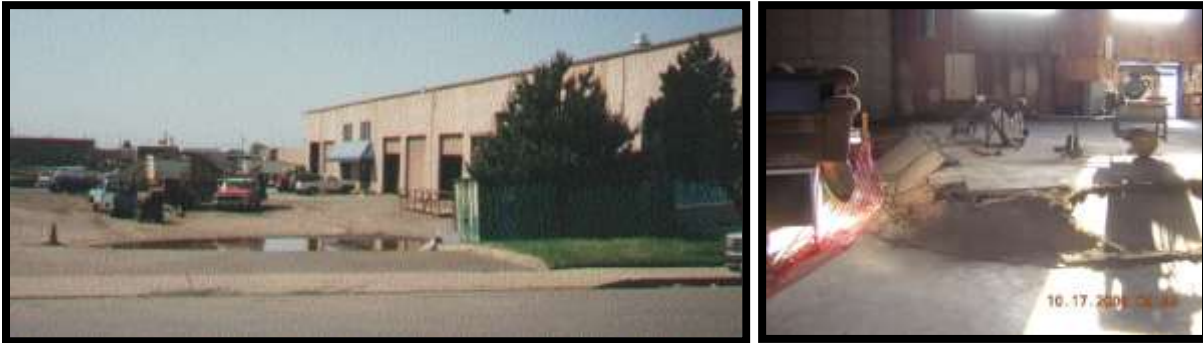
Figure 48: Commercial warehouse at 14 th Avenue (note ponding in parking lot due to settlement); landfill differential settlement damage to warehouse floor (portion of warehouse floor supported by grade beams tied to piles – rest of slab allowed to “float”)
