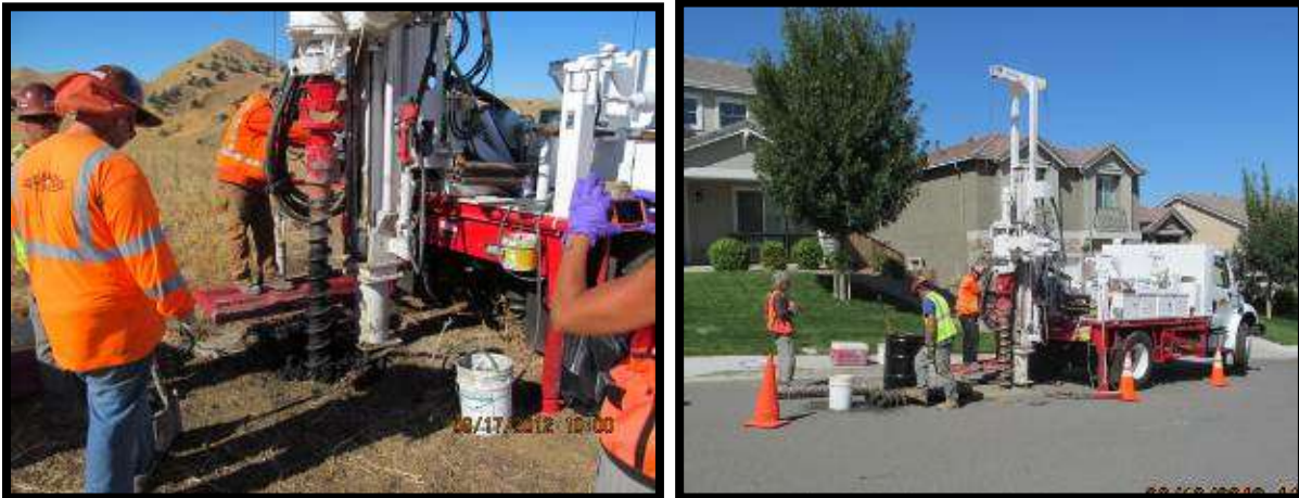
Figure 56: Photo 1: Landfill gas observation well located within the deepest portion of the waste – the bottom elevation of the boring was used to determine the design depth of perimeter monitoring wells; Landfill gas monitoring well installed in the street (Mallard Way) due to a lack of a buffer zone between homes and the boundary of the landfill.
