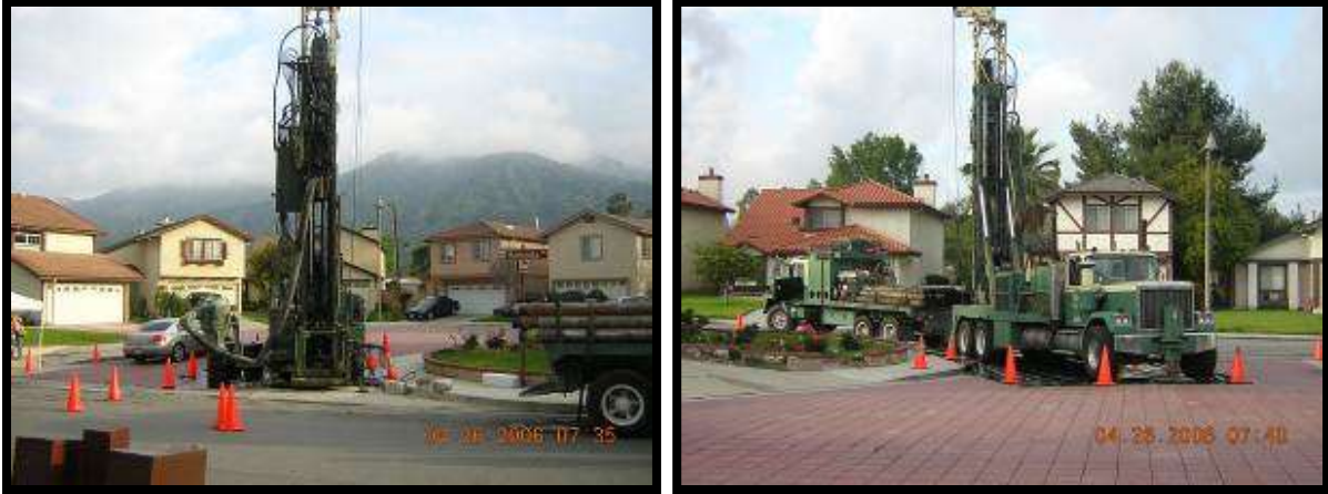
Figure 13: Landfill gas monitoring wells constructed in front of homes adjacent to landfill
