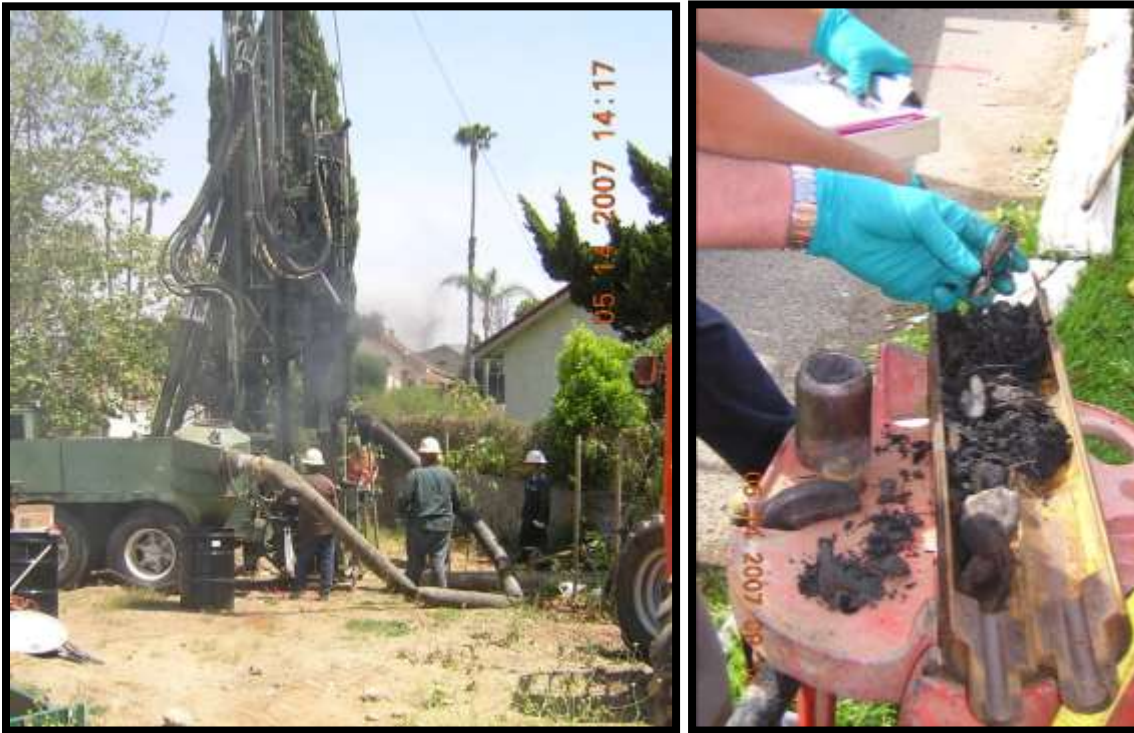
Figure 59: Air percussion drill rig used to construct landfill gas monitoring wells; samples of waste from drilling
