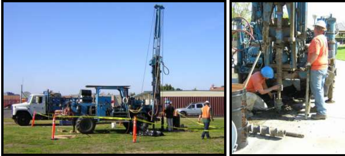
Figure 45: Installation of landfill gas monitoring wells at the Cannery Street Landfill in Orange County
