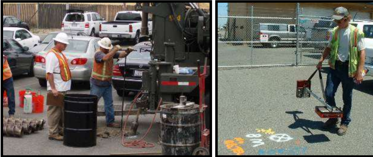
Figure 17: Avoiding damaging unforeseen utilities – hand-augering the first 5 feet; geophysical survey of well location; Call USA
