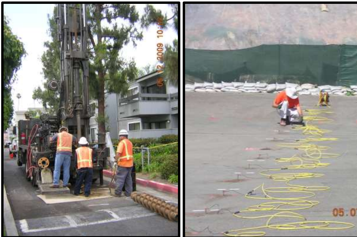
Figure 63: Installation of landfill gas monitoring wells in Westgate Village Apartment Complex; geophysical survey of Rains Pit
