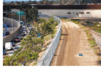
The chain-link fence, in addition to deterring migrants, limits access to a construction canal along the canal, where an elevated highway is being built.
