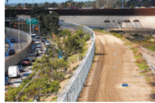
The chain-link fence, in addition to detecting migrants, limits access to a construction zone along the canal, where an elevated highway is being built.
