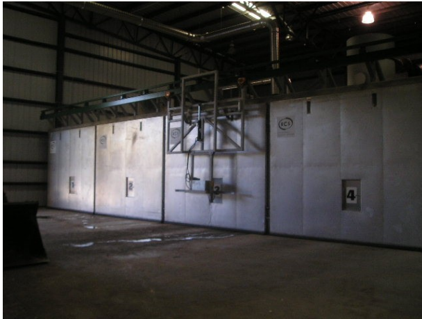
ECS in-vessel compost vessel
