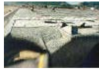
Porous Gas Conductor Under the Concrete Floor
