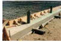
Stand Pipes Located Away from the Building
